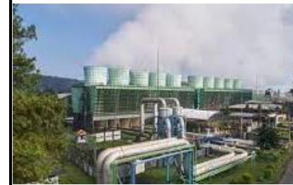
Geothermal Electric Power Station
