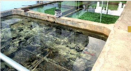
Biological Sedimentation Tank
