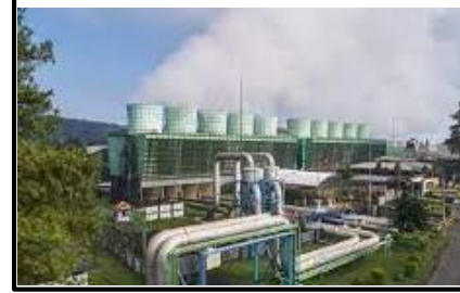
Geothermal Electric Power Station
